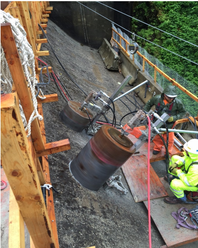
Flashboard Kicker Core Removal
