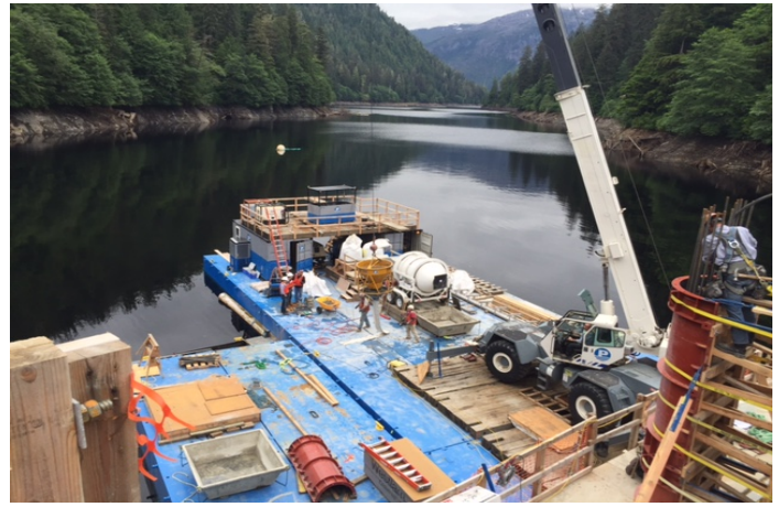
Concrete Batch Plant on Flexi-Float Barge
