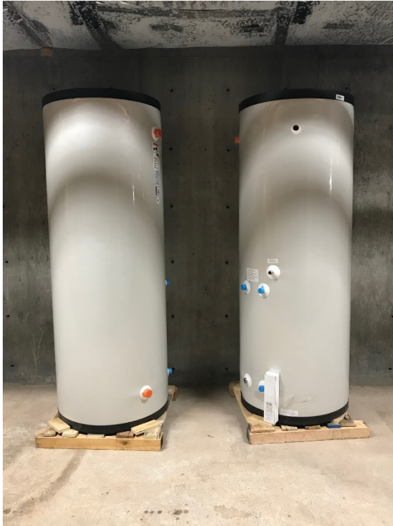
New Hot Water Heaters
