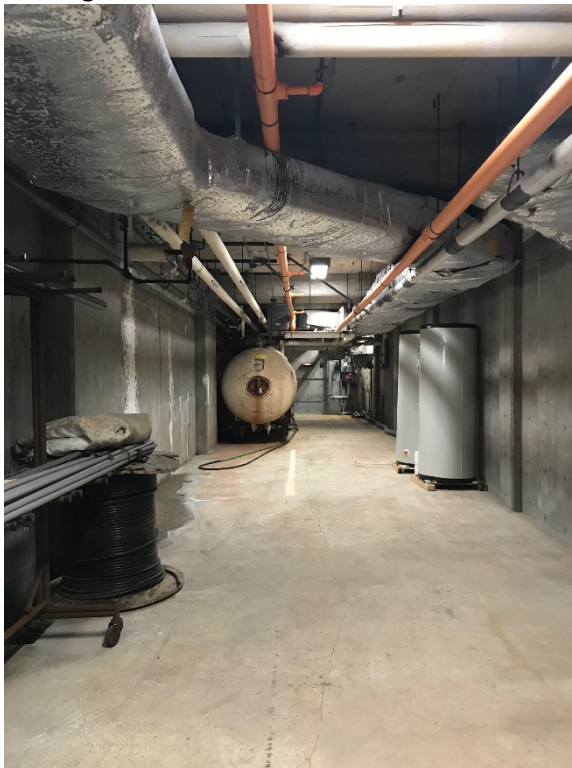
Existing Hot Water Tank – View from end of Corridor where it will be relocated
