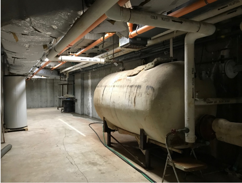
Existing Hot Water Tank – View to the far end of the Corridor where it will be relocated
