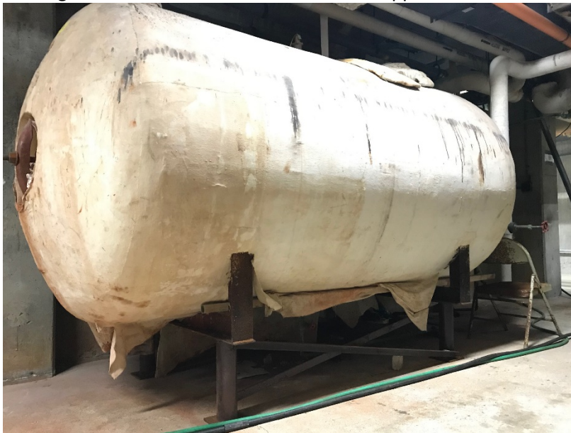
Existing Hot Water Tank – View of tank and support
