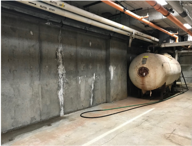
Existing Hot Water Tank – Closer view from end of Corridor where it will be relocated
