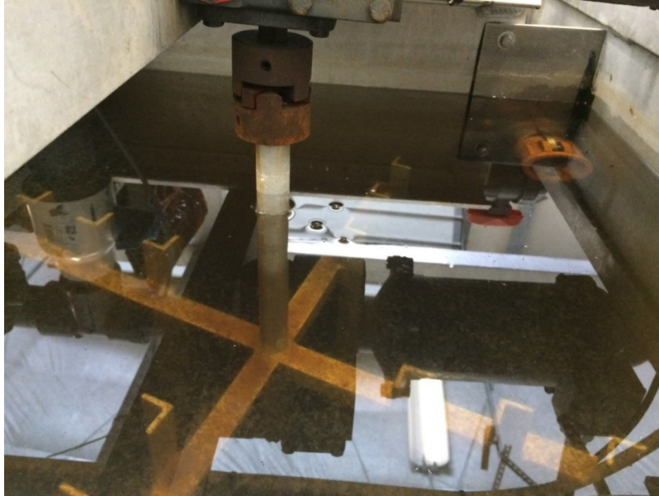
Figure 5 - Pilot Plant Flocculation Basin
