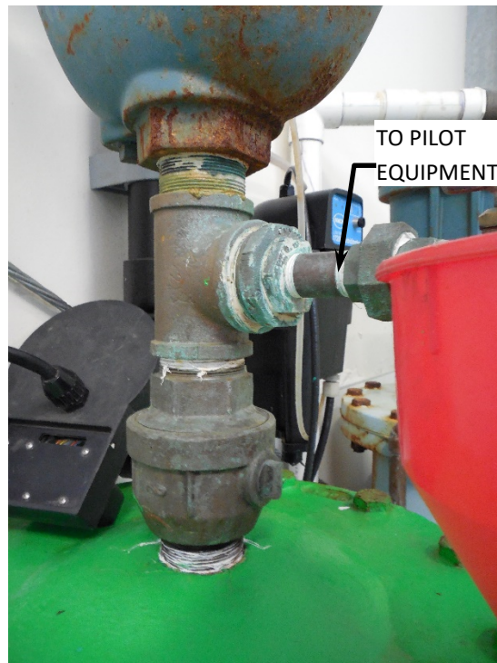
Figure 2 - Raw Water Connection
