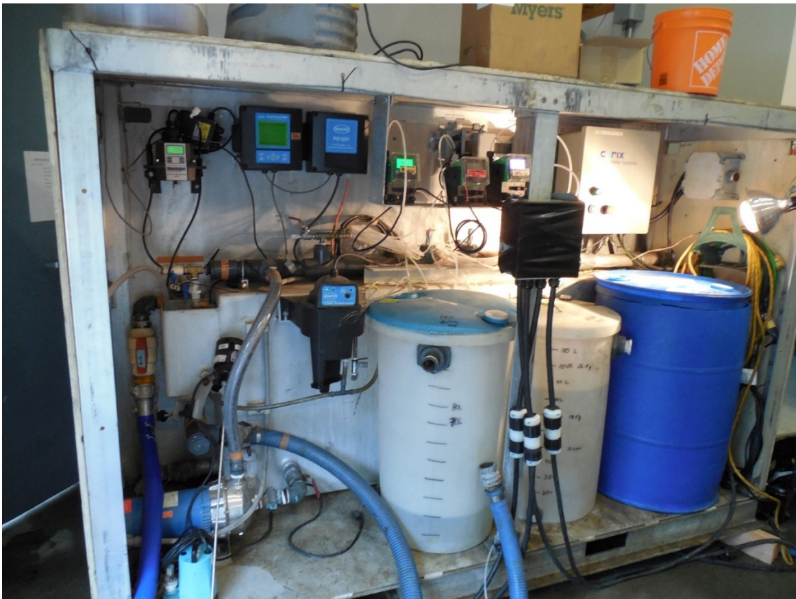
Figure 4 - Pilot Plant Chemical Injection Equipment
