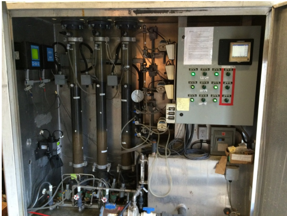
Figure 8 - Pilot Plant Control Panel and Multimedia Filters
