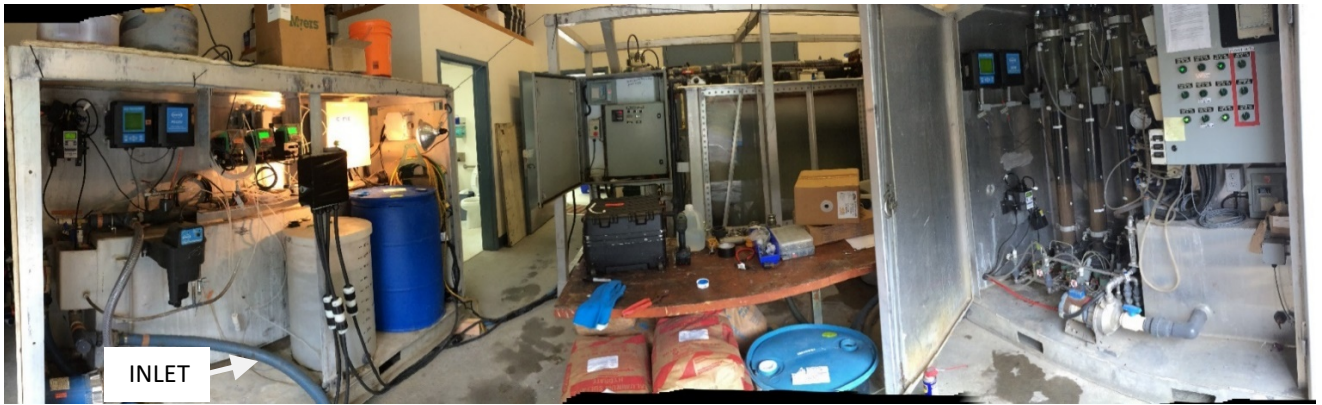
Figure 10 Pilot Plant Overview
