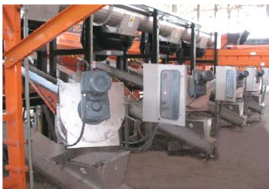
4 ÖÜÿÔÇÖÁÜÒÙ units positioned in parallel providing sludge dewatering from 1.6% DS to 20% DS
