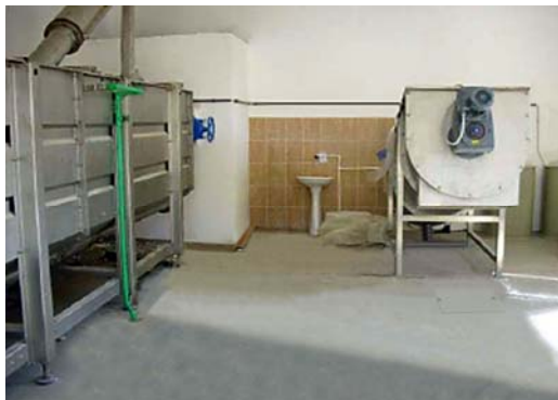
XMD 70 ÖÜÿÔCSÒÁÛÜÒÙÙ with TOP 3 Combined Screen, Grit and FOG removal plant installed inside a purpose-built building
