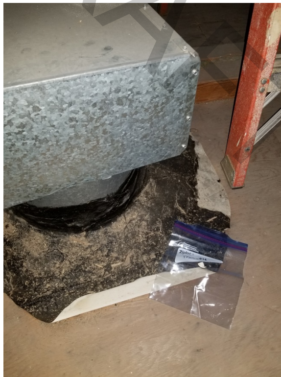
Photo 2: Tar paper skirts around penetrations in the new portion of the attic are ACM. (May 23, 2018)
