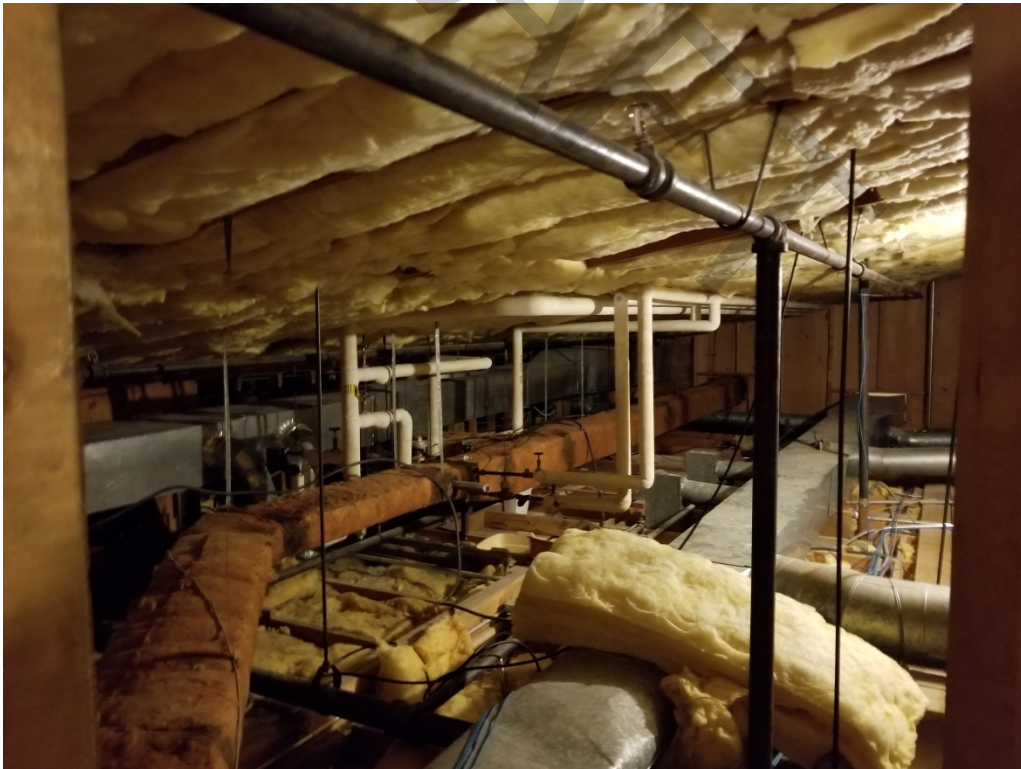
Photo 14: Presumed ACM TSI in the attic under the roof of the original building. (May 22, 2018)
