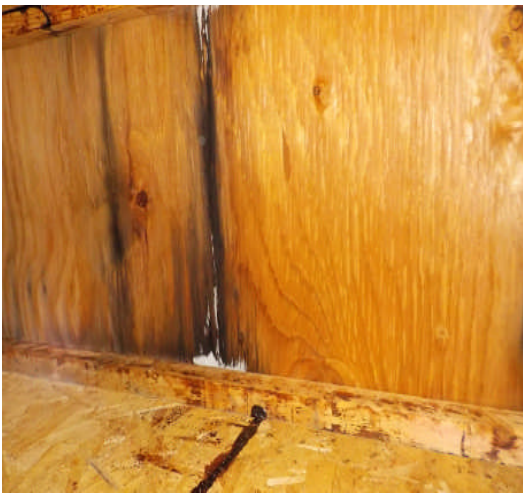
Deficiency Item S01. Minor roof leak creating moist condition for mildew growth (white).
