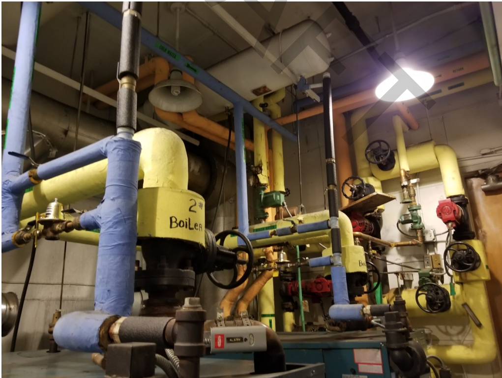
Photo 12: Presumed ACM TSI in the boiler room. Flue in back corner is assumed to contain ACM insulation. (May 22, 2018)
