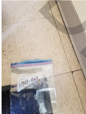
Photo 6: Off-white floor tiles in the stairway were ACM, and had a black mastic with trace amounts of asbestos. (May 22, 2018)
