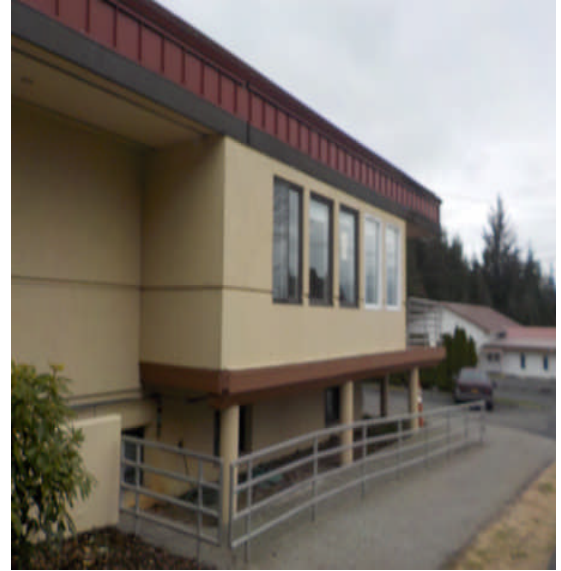
Deficiency Item S16. Addition bump out to activities room. Water runs down beneath the wall sole plate and runs across the floor. Foundation piers have settled.
