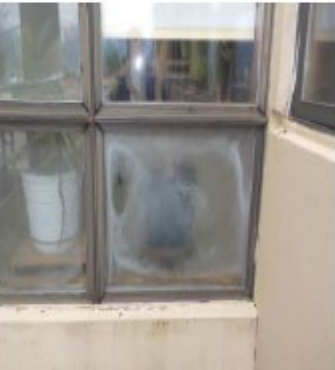
Deficiency Items S06, S07 and S08. Example damaged EIFS (freeze-thaw), fogged window, caulking sealant failure, siding in need of exterior paint
