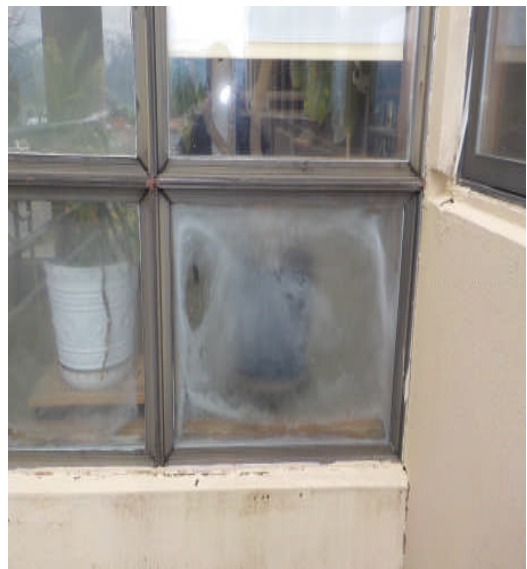
Deficiency Items S06, S07 and S08. Example damaged EIFS (freeze-thaw), fogged window, caulking sealant failure, siding in need of exterior paint
