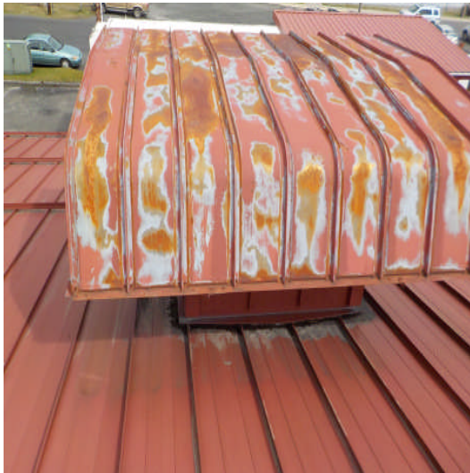
Deficiency Item S03. Air handler hood with corrosion.
