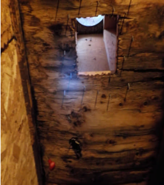
Deficiency Item S01. Decayed plywood roof sheathing typical at (2) roof ventilation turrets. Nontypical condition of framing.
