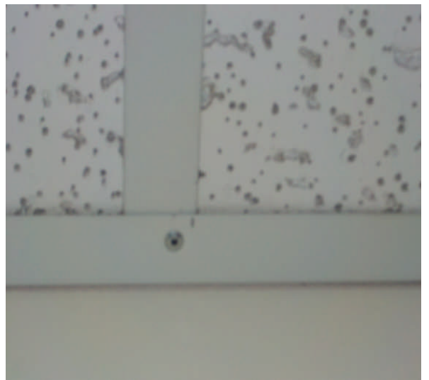
Deficiency Item S12. Rooms over 144 sf, metal grid runners are fastened to angle on all four sides of ceiling. Only one side shown in photo.
