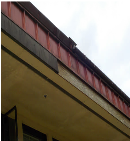
Deficiency Item S05. Missing EIFS fascia.
