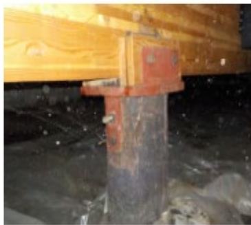
Typical creosote treated timber piling beneath 1988 addition, below emergency room. In good condition.
