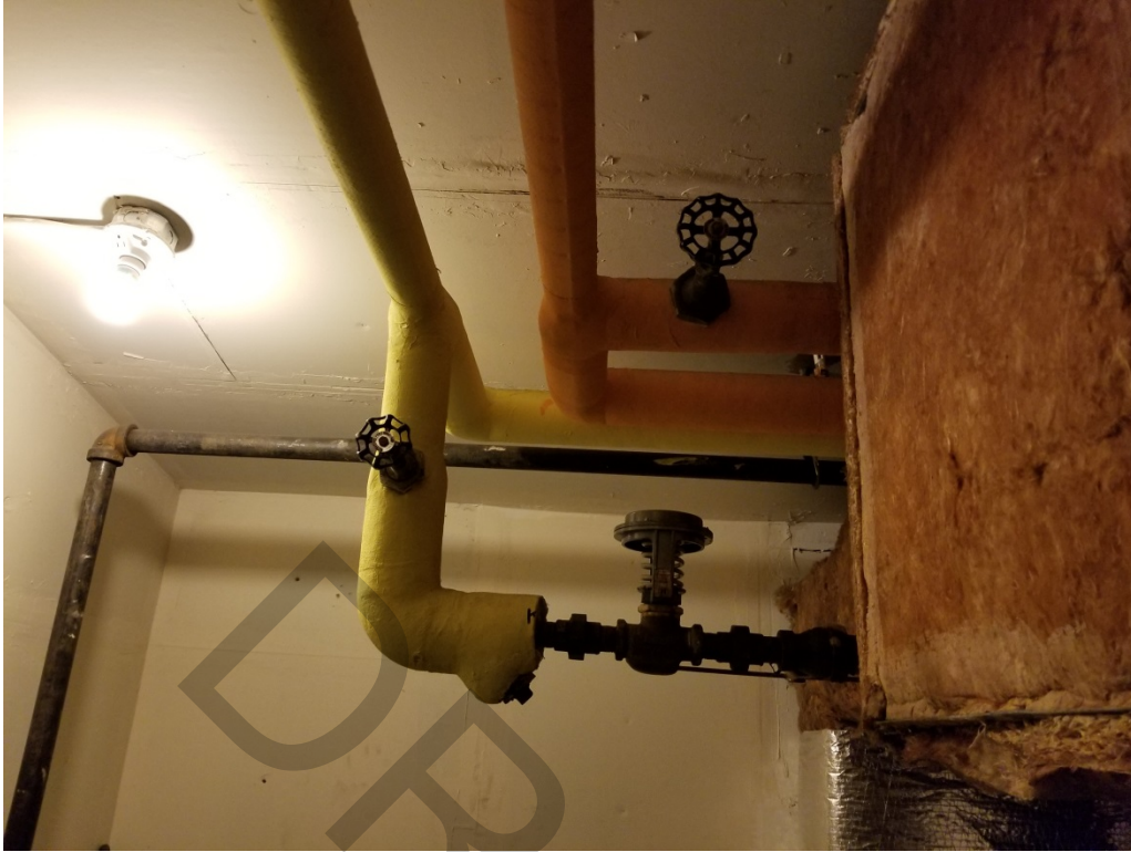
Photo 13: Presumed ACM TSI in the air handler room. Orange duct insulation on the right is not ACM. (May 22, 2018)
