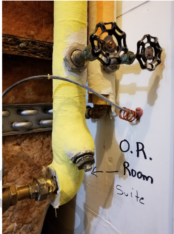
Photo 15: Exposed ends of presumed ACM TSI hard insulated joints. (May 22, 2018)
