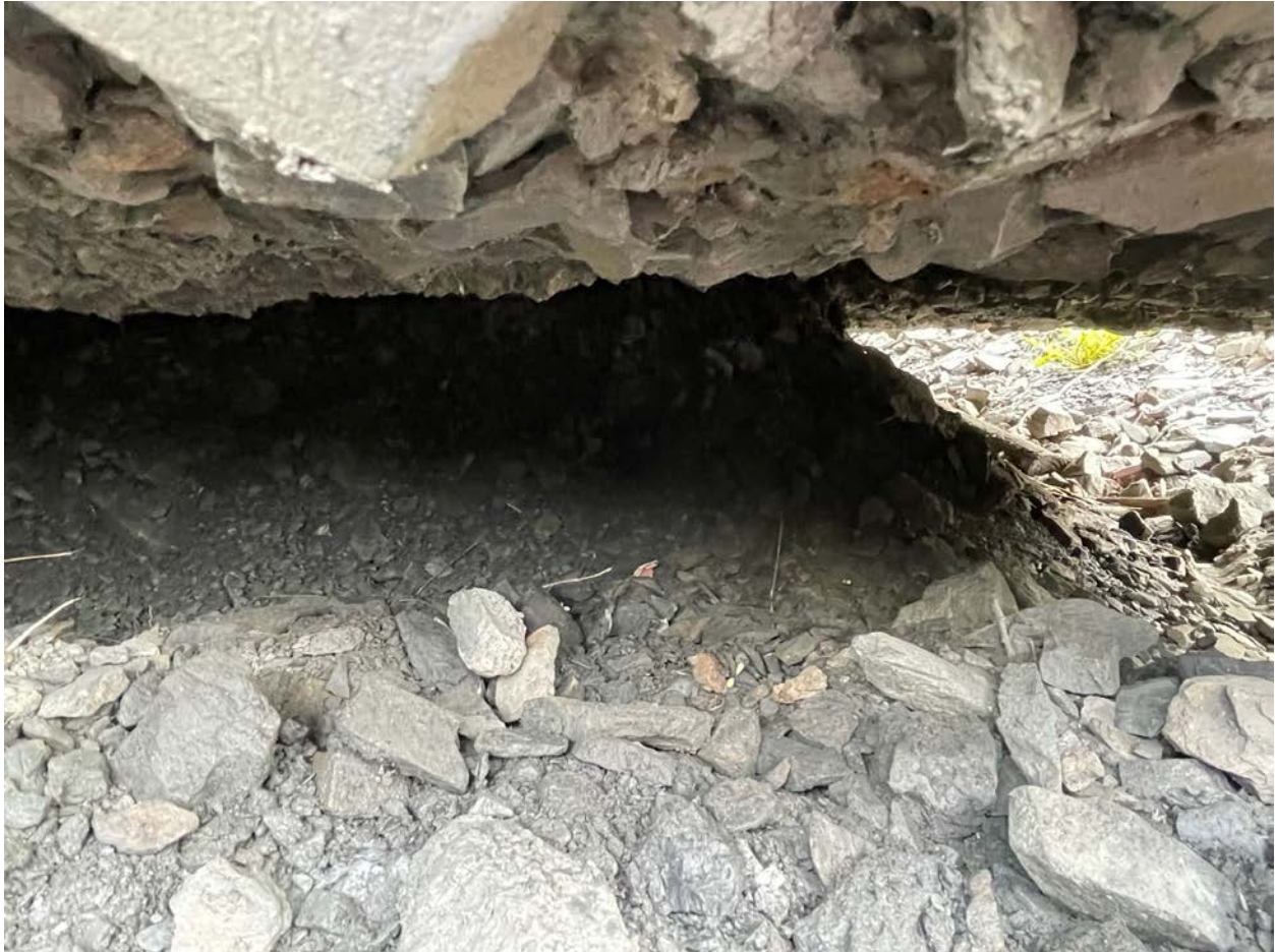
Void Under Slab at Southwest Corner of Building
