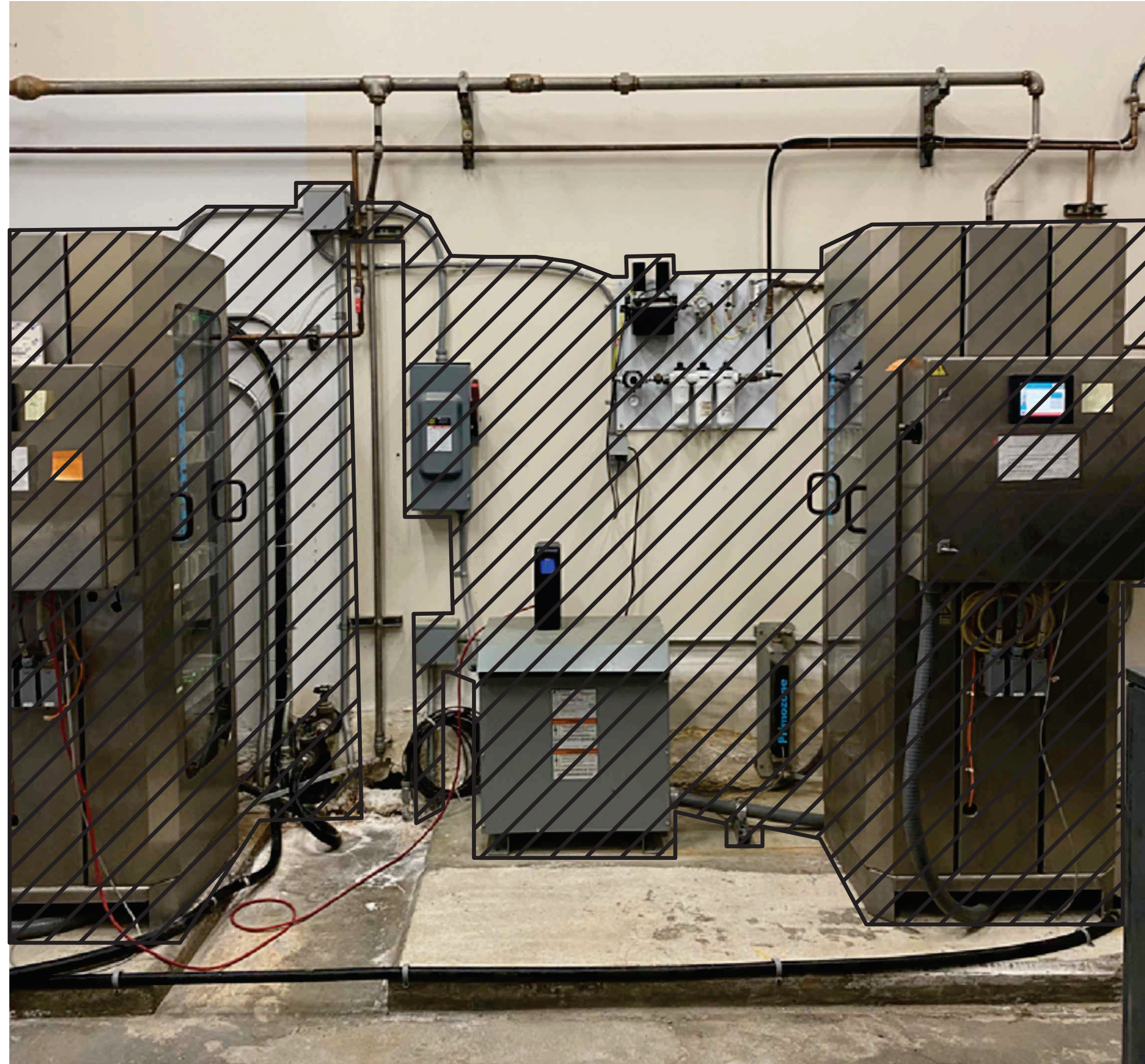
1 ADMIN BUILDING OZONE ELECTRICAL EQUIPMENT (DEMOLISH)
