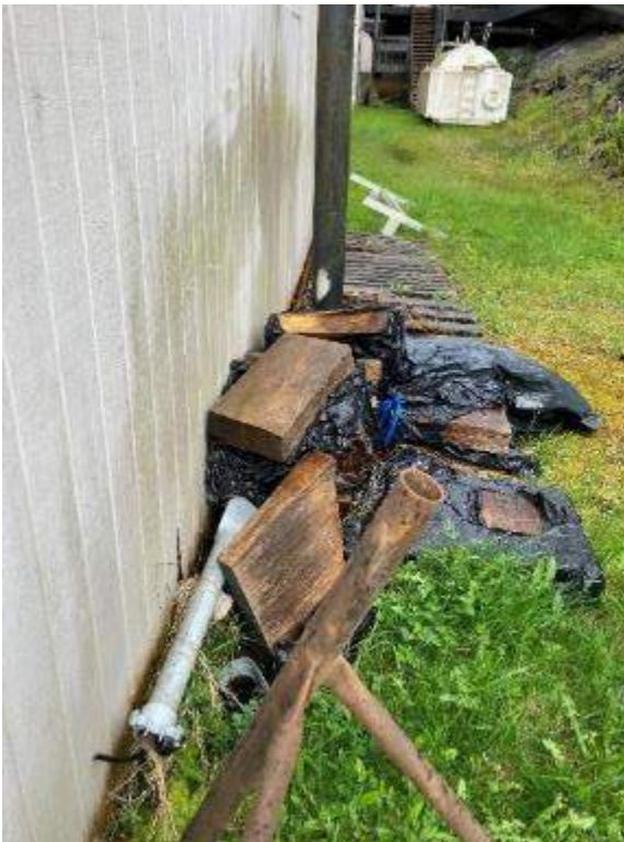
Materials stored against exterior wall
