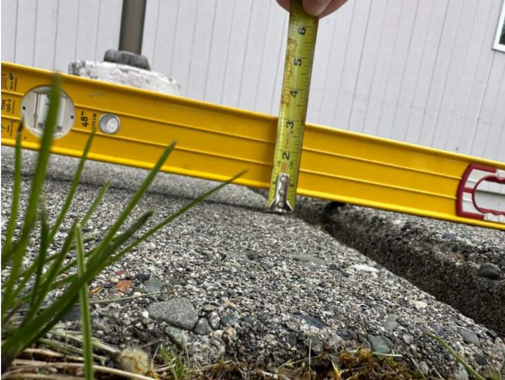
Abrupt drop between panels in sidewalk on southwest side of building, top level
