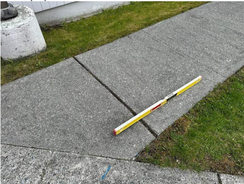
Wide gap between panels in sidewalk on southwest side of building, top level
