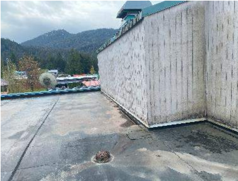
Siding in poor condition at mechanical penthouse
