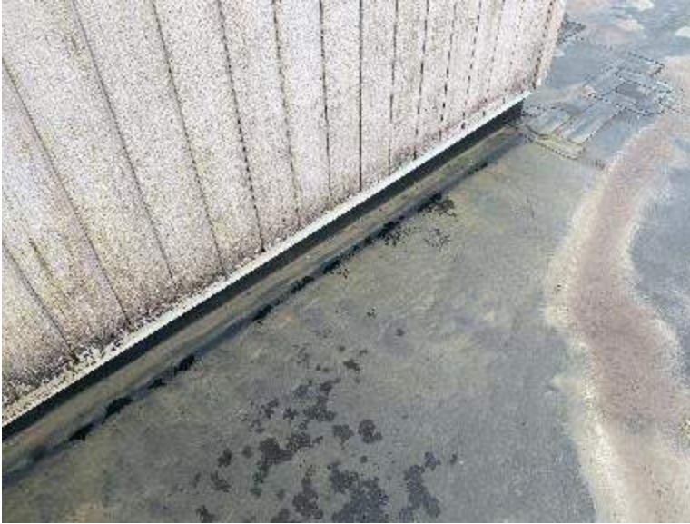
Water intrusion behind siding
