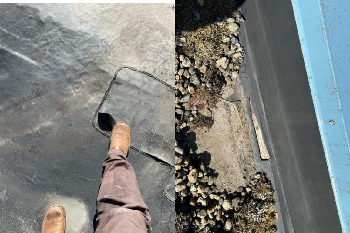
Delam and water-swelling OSB visible
