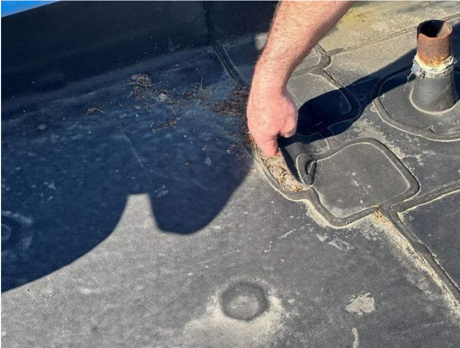
Delaminating laps in 1995 roof.
