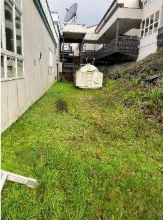
Standing water on the north side of the building
