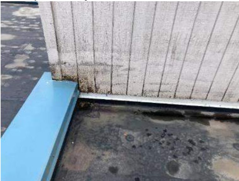
Rotten siding at base of mechanical penthouse wall
