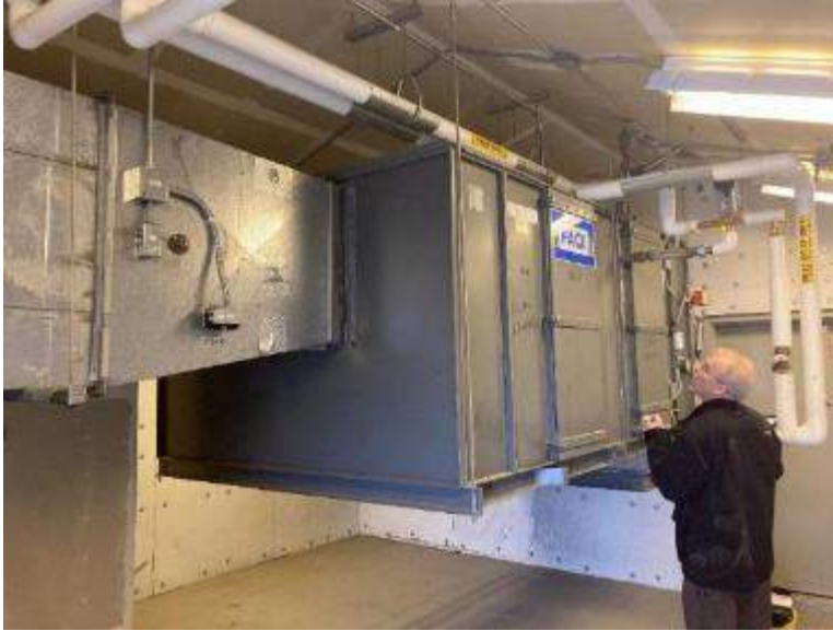
Suspended mechanical not seismically braced
