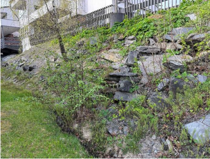
Saturation and standing water in vegetated area northeast of vocational wing
