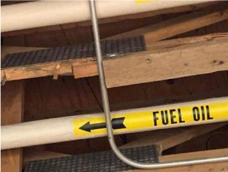
Damaged bottom chord of floor truss
