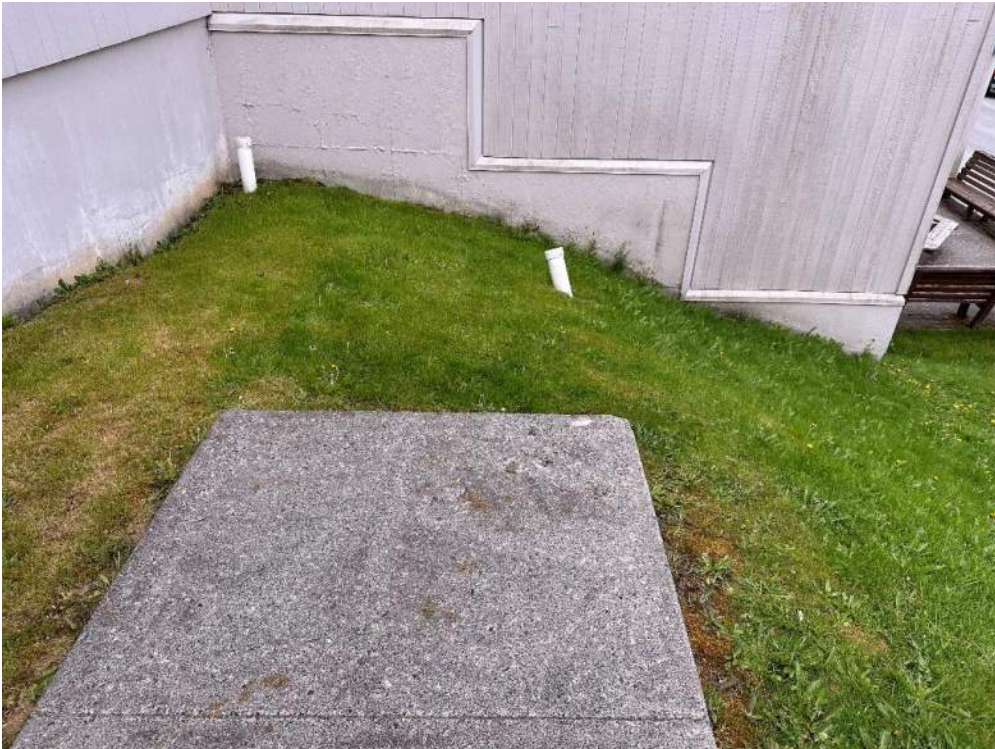
Sidewalk on southwest side of building, top level, ends abruptly near steep slope
