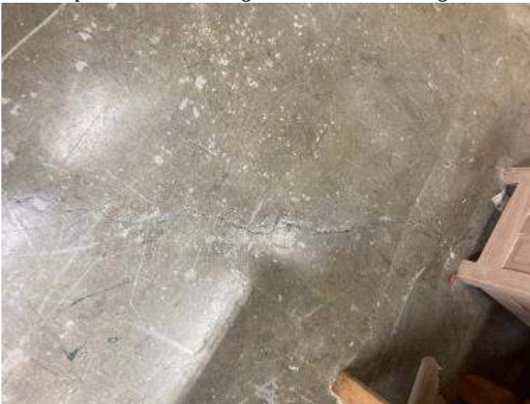
Crack in slab-on-grade in shop
