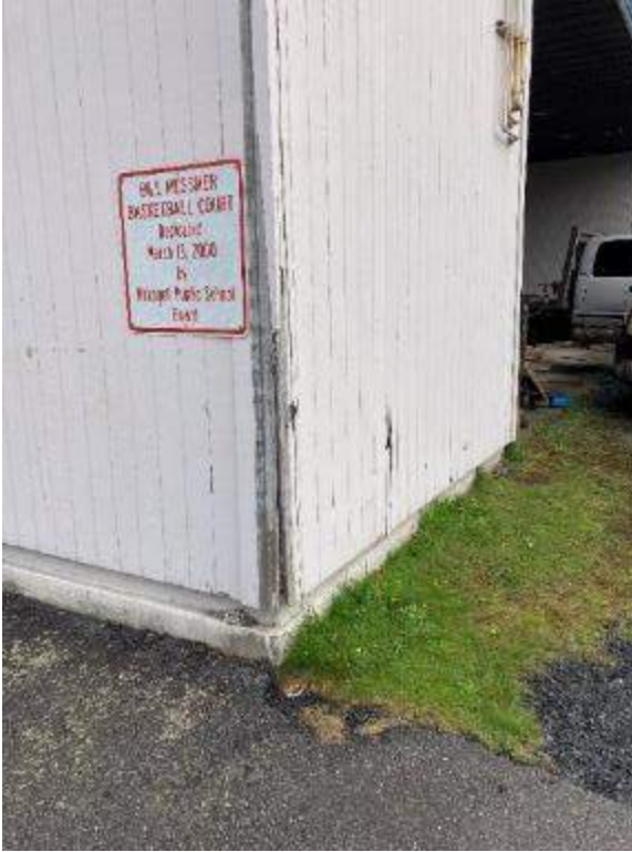
Vehicular damage to exterior wall
