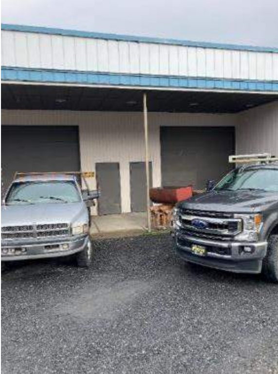
Unprotected exterior column
