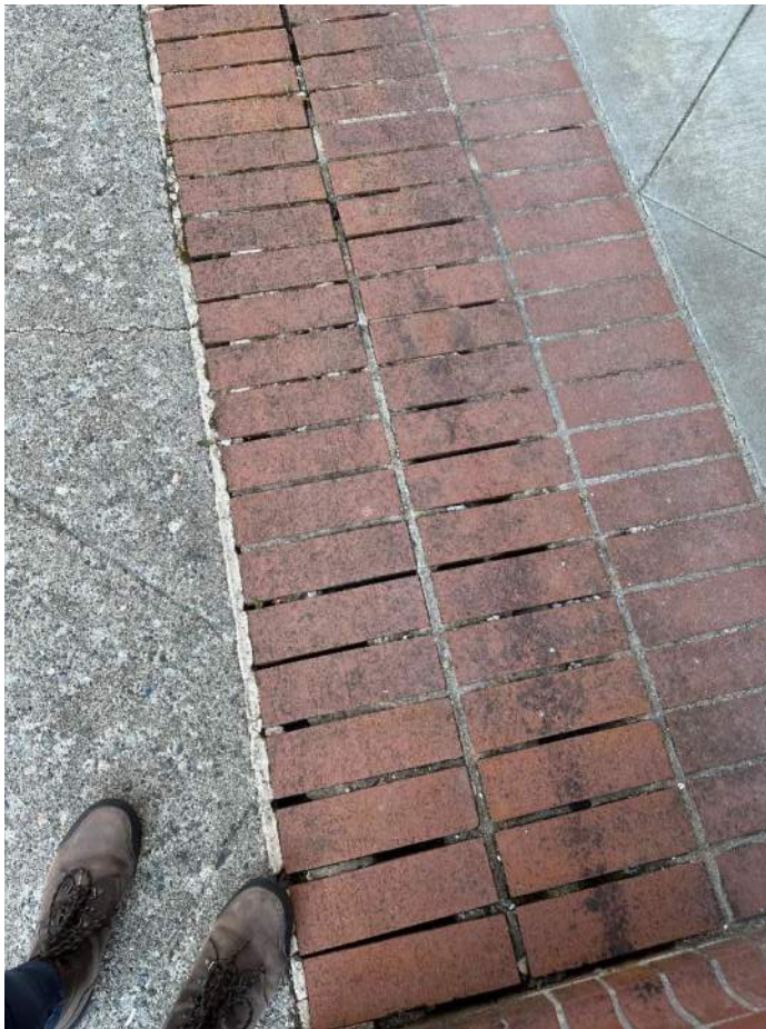
Hardscape brick-work to be repointed.
