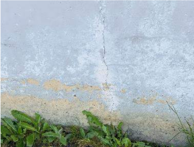
Crack in foundation wall
