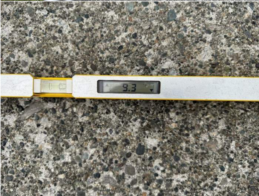
Location where access ramp longitudinal slope exceeds the ADA maximum
