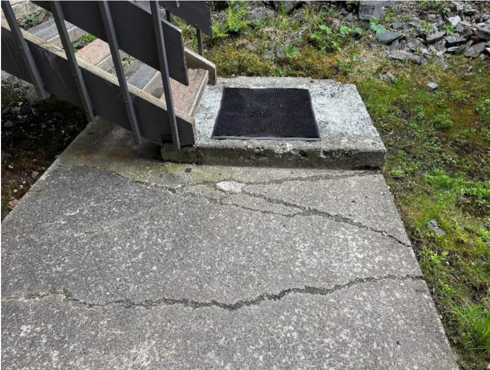
Replace concrete apron at base of stairs leading down from breezeway
