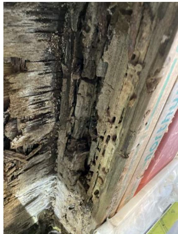
Photo 12a – Dry rot and carpenter ant damage at base of exterior wall
