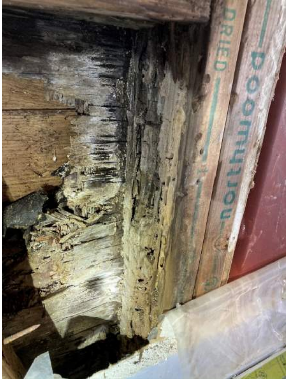
Photo 12b – Dry rot and carpenter ant damage at base of exterior wall
