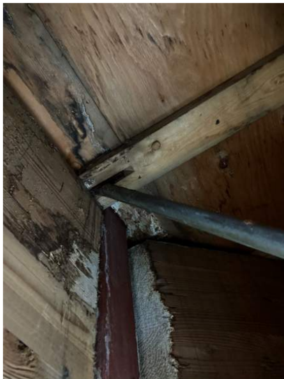
Photo 8 – Water stains on floor sheathing and glu-lam beams at exterior wall at Level 2 floor
