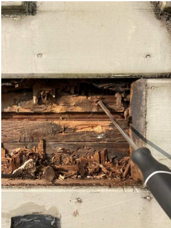
Photo 7a – Dry rot in exterior wall at Level 2 floor
