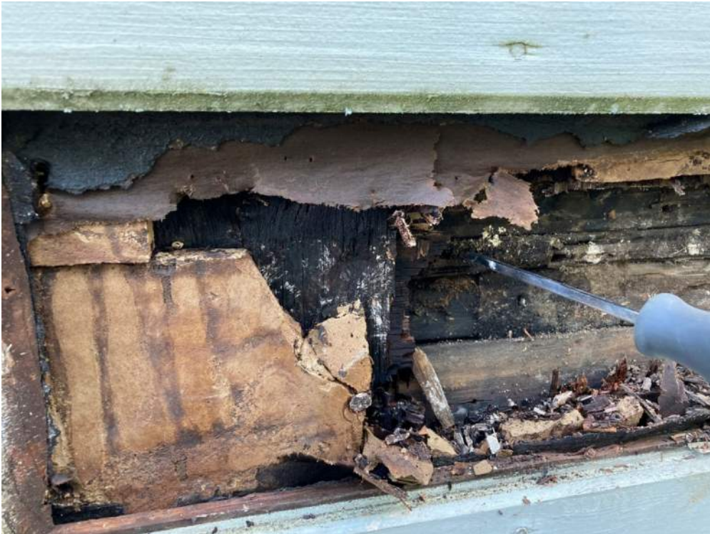
Photo 14b – Rot in exterior wall at Level 2 floor
