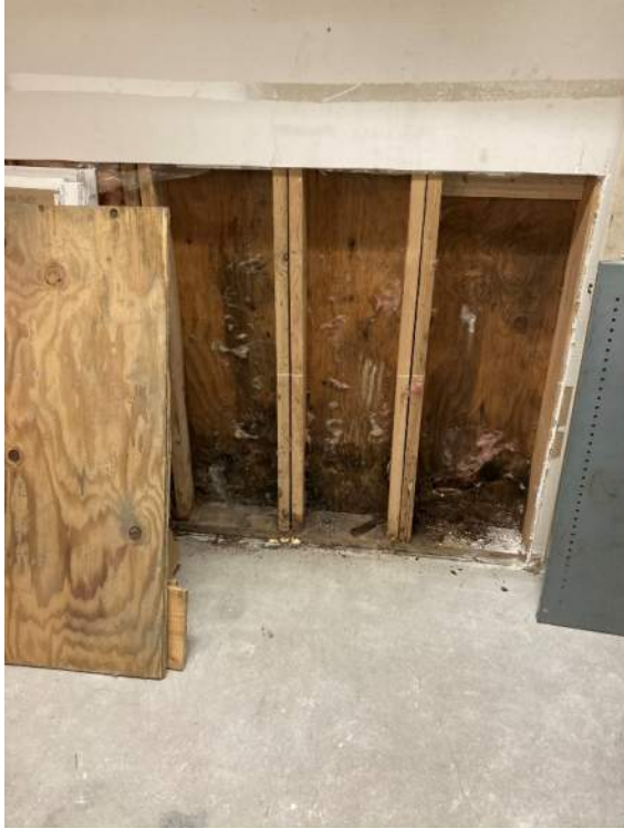
Photo 5a – Deterioration at base of exterior wall
