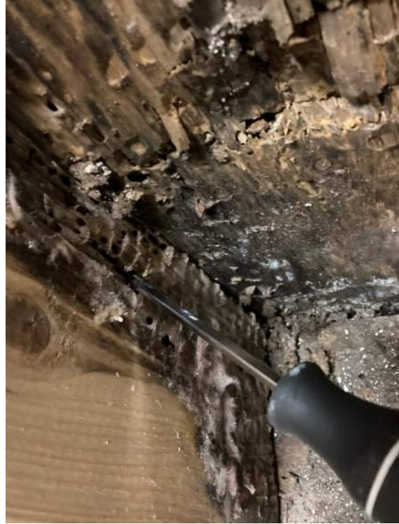
Photo 5b – Dry rot and carpenter ant damage at base of exterior wall
