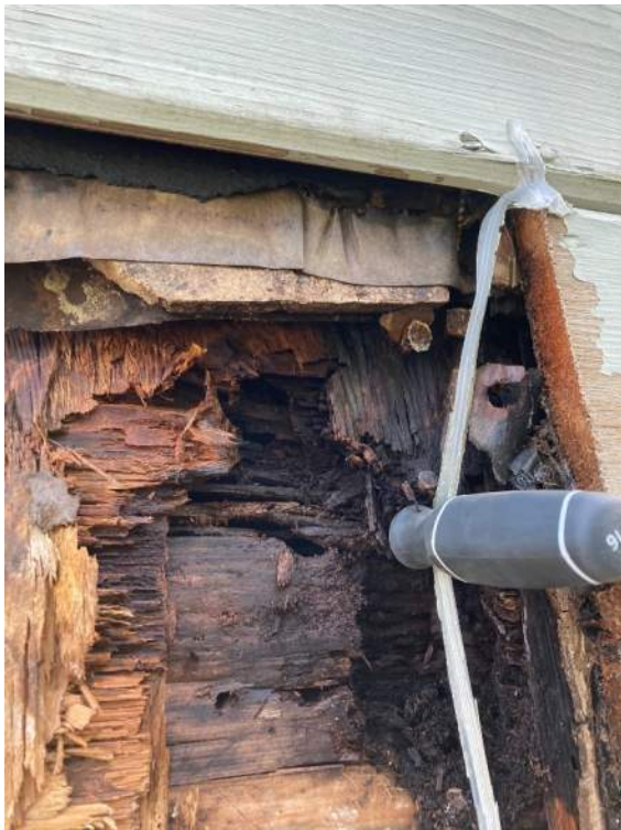
Photo 23b – Rot in exterior wall at roof
