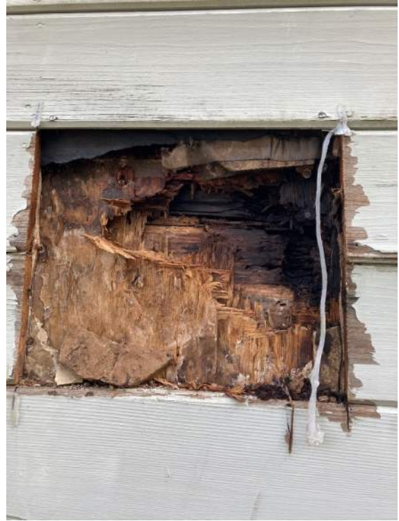
Photo 23a – Rot in exterior wall at roof
