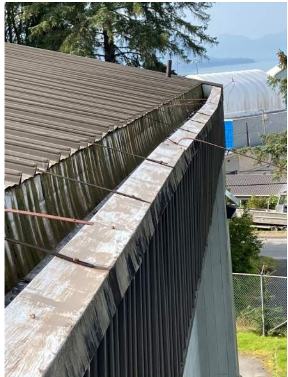
Photo 28 – Deflection of gutter and broken straps
