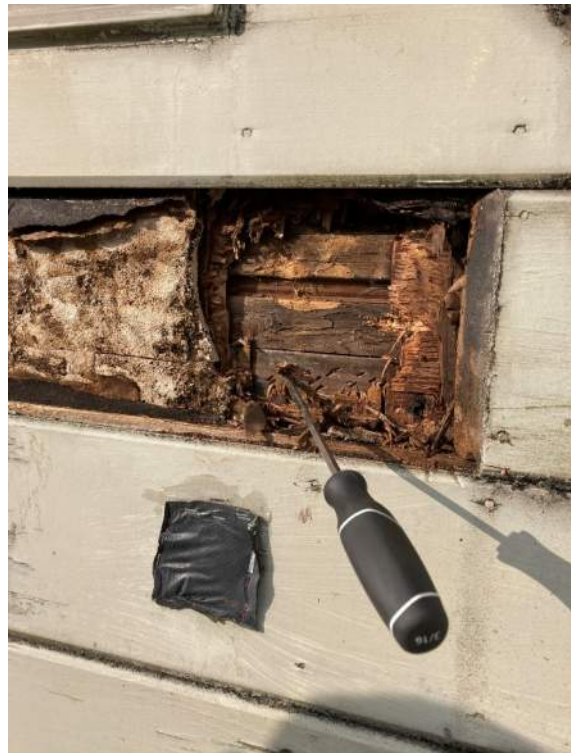
Photo 7b – Dry rot in exterior wall at Level 2 floor
