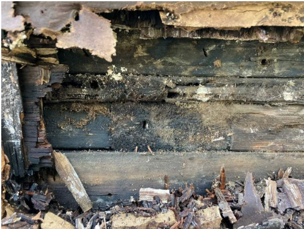
Photo 14d – Rot in exterior wall at Level 2 floor
