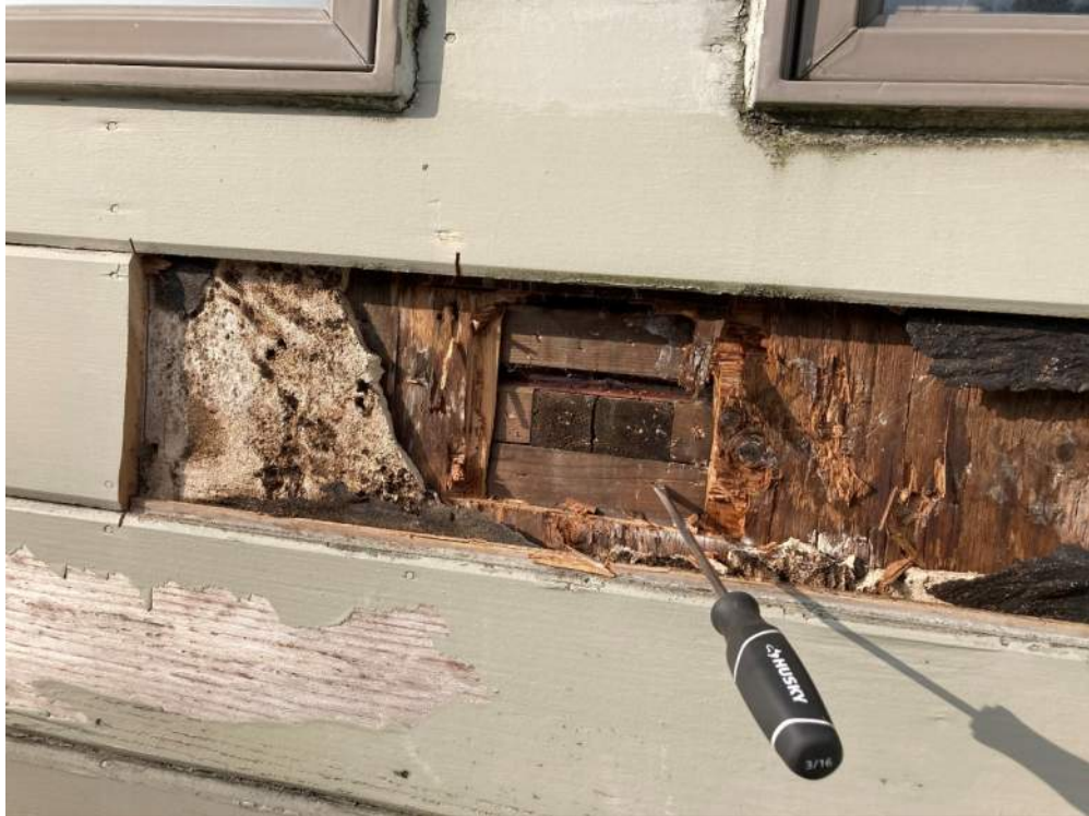
Photo 7c – Dry rot in exterior wall at Level 2 floor
