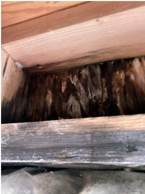
Photo 13 – Deterioration at exterior soffit at Level 2
