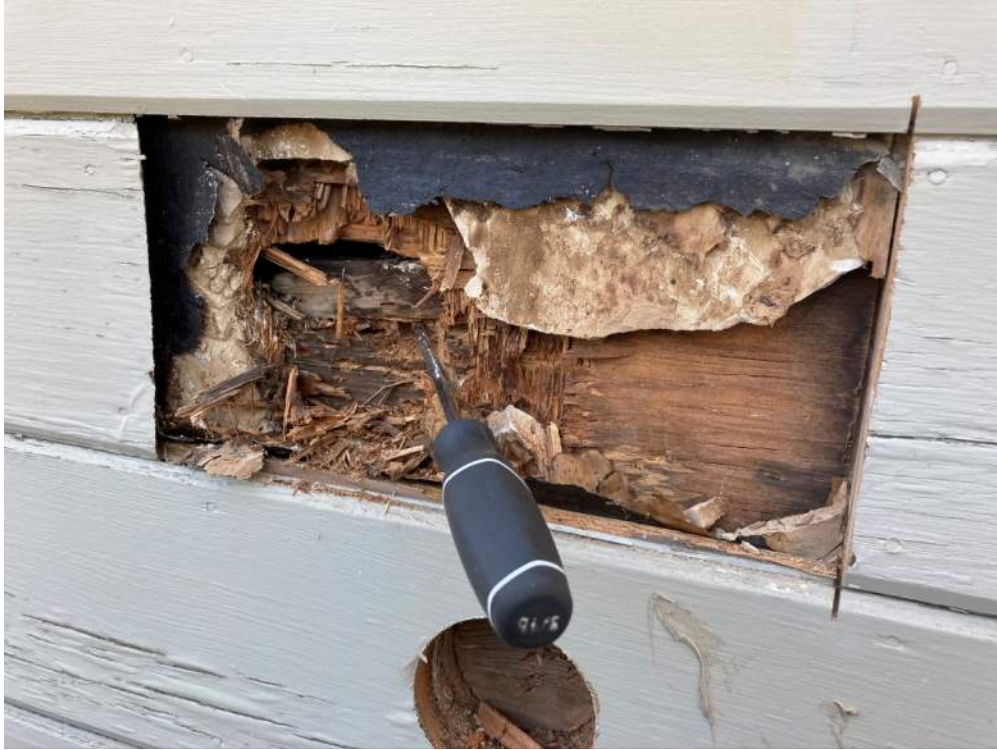
Photo 16 – Dry rot in exterior wall at roof
