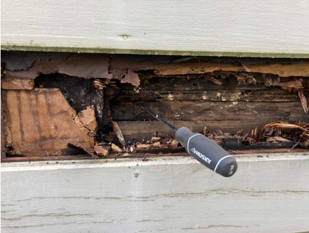
Photo 14a – Rot in exterior wall at Level 2 floor
