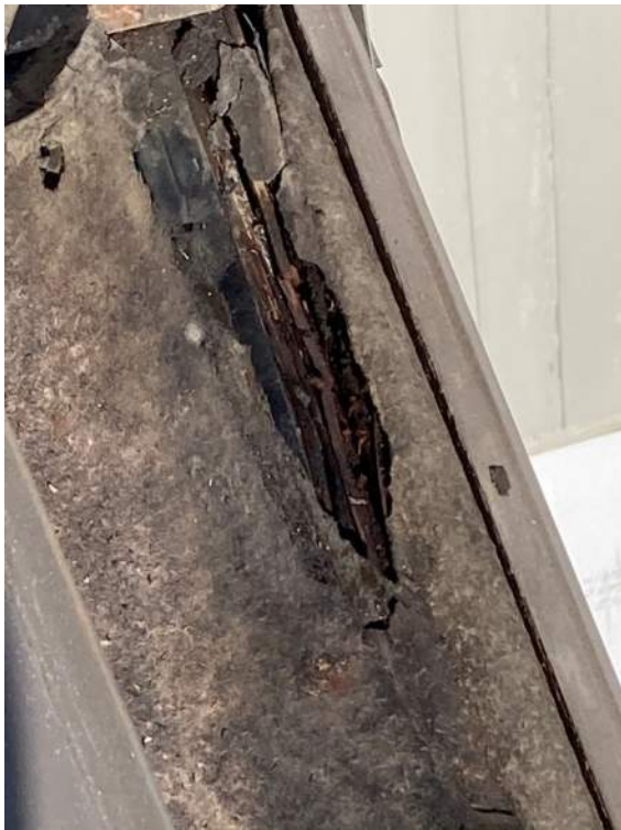
Photo 17 – Rot in exterior wall parapet
