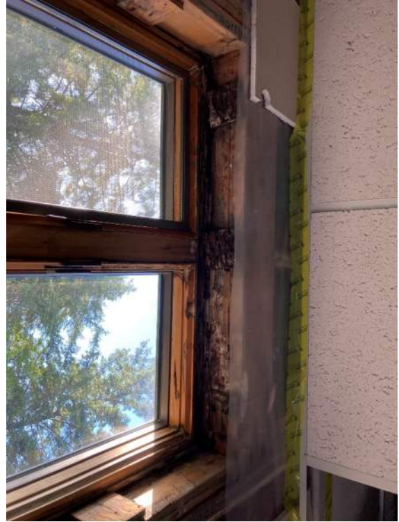
Photo 12c – Deterioration at window in exterior wall
