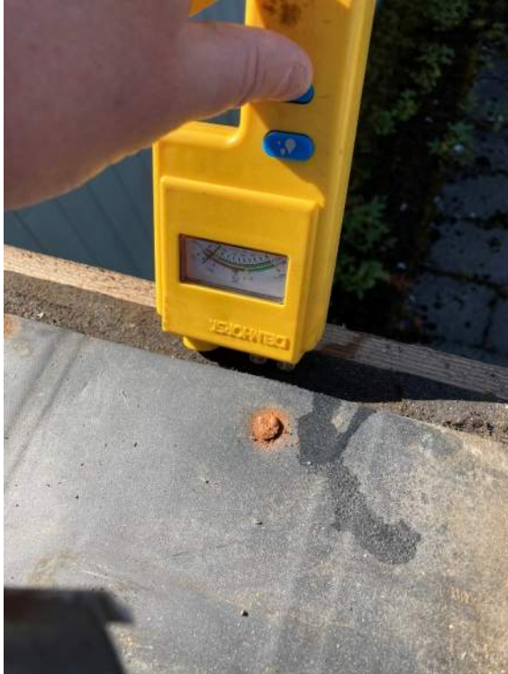
Photo 31 – Excessive moisture in exterior wall parapet
