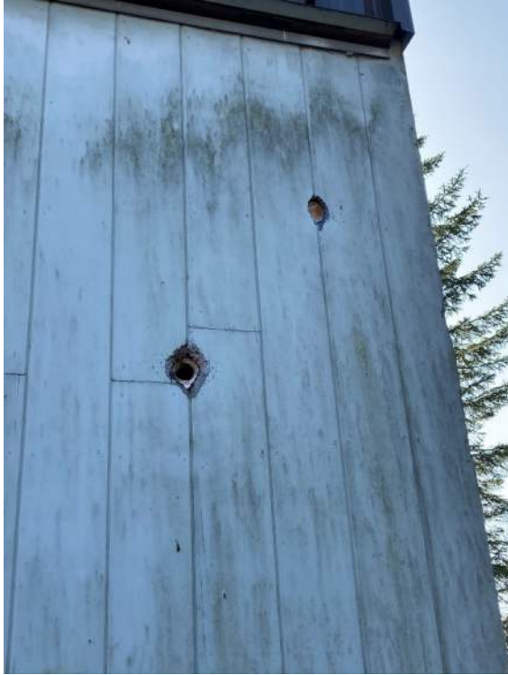
Photo 21 – Woodpecker holes in exterior wall
