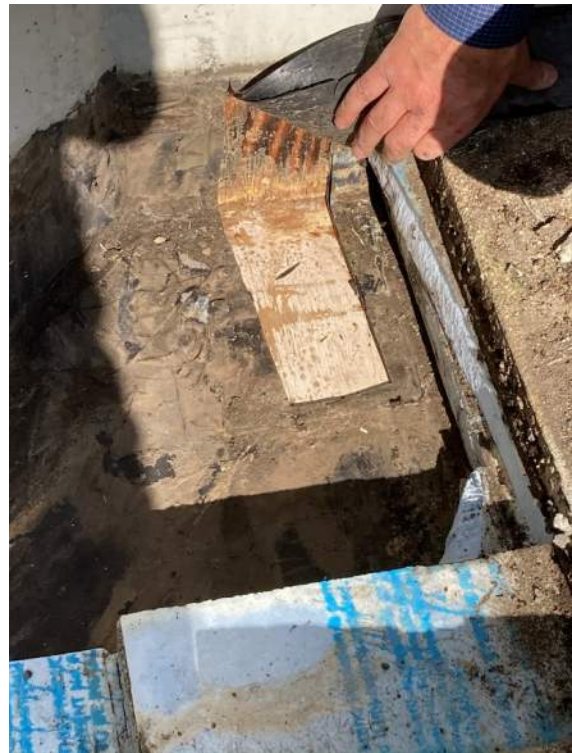
Photo 18 – Damp wall sheathing and roof plywood
