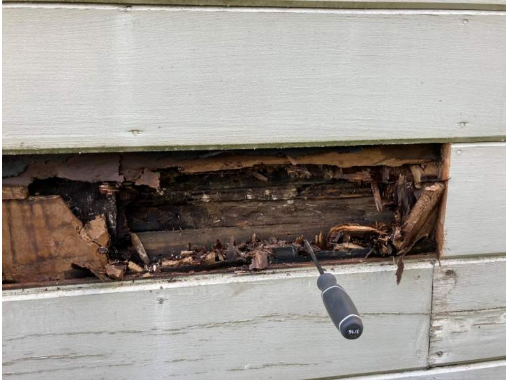
Photo 14c – Rot in exterior wall at Level 2 floor
