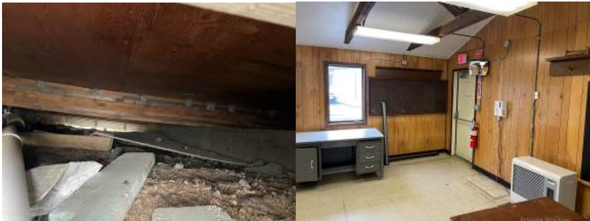
Above left is the underside of the building and as can be seen the subject is sitting on wood grade beams. Above right is a view of the interior looking at the NE corner. The oil fired Toyo heater is viewers right.
