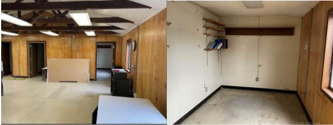
Pictured above left is the main hall which can be used for larger gatherings. Pictured right is an office with an outside window.
