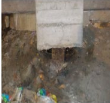
Typical creosote treated timber piling beneath 1968 Construction, beneath kitchen. In good condition. Reinforced concrete pile cap and grade beams in good condition.
