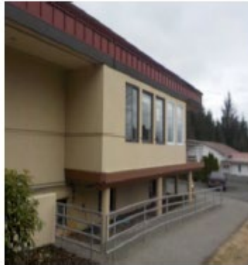
Deficiency Item S16. Addition bump out to activities room. Water runs down beneath the wall sole plate and runs across the floor. Foundation piers have settled.
