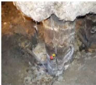
Deficiency Item S17. Decayed creosote treated timber piling. Nontypical condition, not representative of average piling condition. Most pilings were found to be in good condition.
