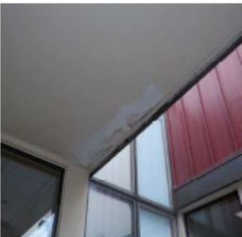
Deficiency Item S04. Example water damaged roof soffit sheathing.
