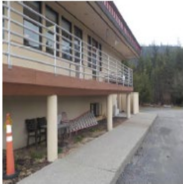
Deficiency Item S15. Note dip in deck rim board. Guardrails non-code compliant. Space between horizontal rails exceeds 4". Connection to deck not capable or resisting a force of 200 pounds.
