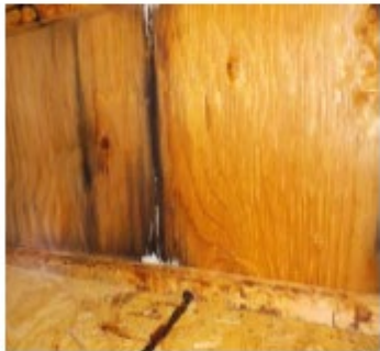
Deficiency Item S01. Minor roof leak creating moist condition for mildew growth (white).
