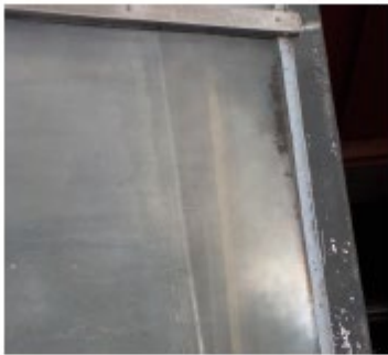
Deficiency Item S09. Broken skylight glazing.
