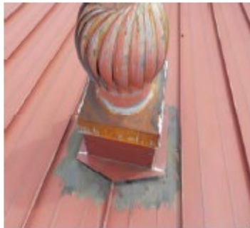
Deficiency Item S01. Example roof ventilation turret above major roof leak.
