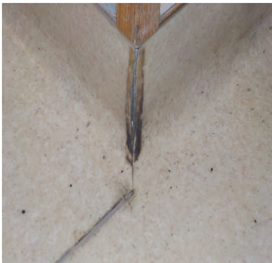
Deficiency Item S11. Example vinyl Flooring seam failure.
