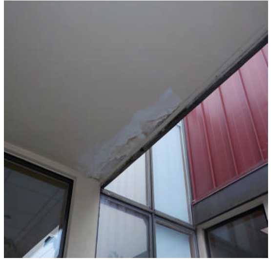
Deficiency Item S04. Example water damaged roof soffit sheathing.
