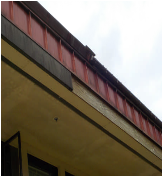
Deficiency Item S05. Missing EIFS fascia.
