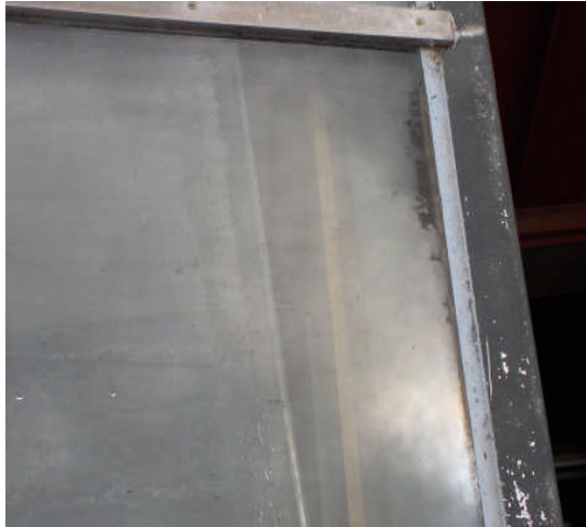
Deficiency Item S09. Broken skylight glazing.
