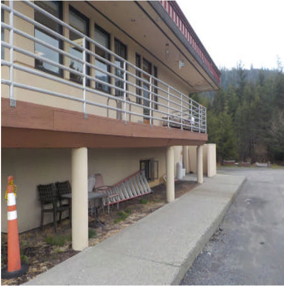
Deficiency Item S15. Note dip in deck rim board. Guardrails non-code compliant. Space between horizontal rails exceeds 4". Connection to deck not capable or resisting a force of 200 pounds.
