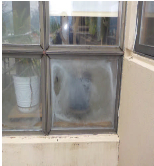
Deficiency Items S06, S07 and S08. Example damaged EIFS (freeze-thaw), fogged window, caulking sealant failure, siding in need of exterior paint
