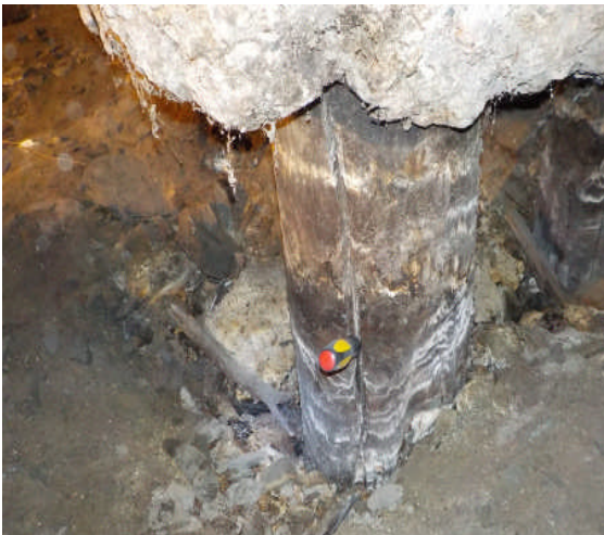
Deficiency Item S17. Decayed creosote treated timber piling. Nontypical condition, not representative of average piling condition. Most pilings were found to be in good condition.
