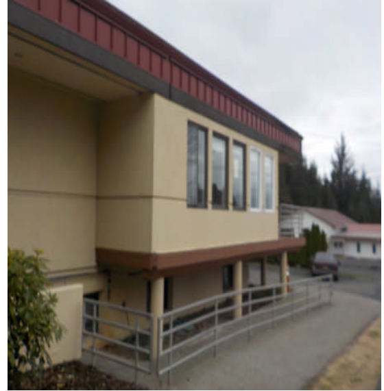
Deficiency Item S16. Addition bump out to activities room. Water runs down beneath the wall sole plate and runs across the floor. Foundation piers have settled.
