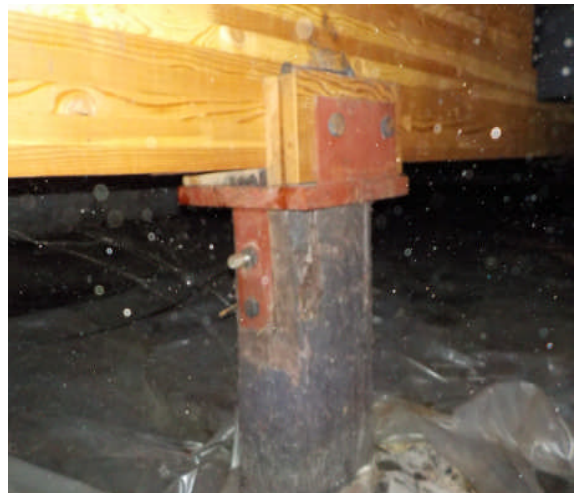
Typical creosote treated timber piling beneath 1988 addition, below emergency room. In good condition.
