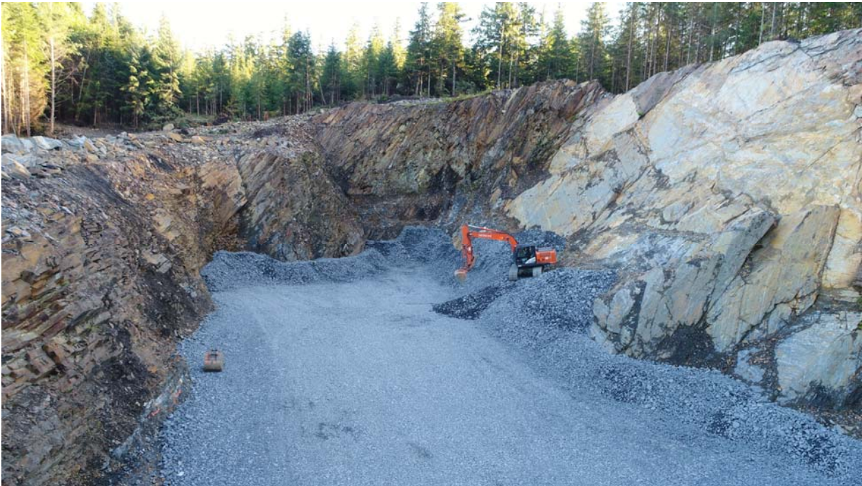
Photo 1: Monofill Site, September 13, 2016. 6" rock for Base Drain is installed, beginning of Chimney Drain
