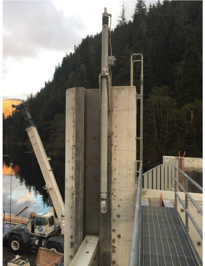
Hydraulic gate actuator - center pier
