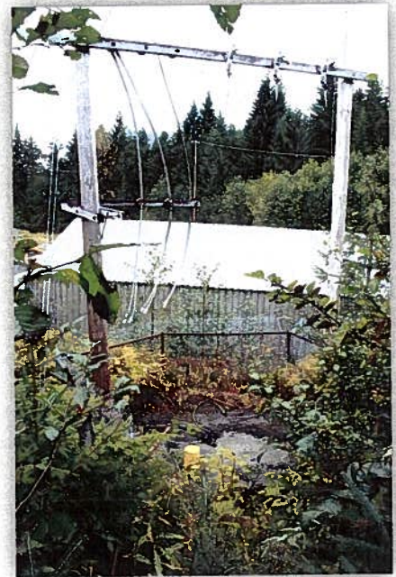
Figure 11: City-Tie Transformer Pad
