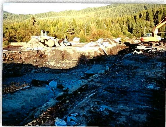
Figure 14: July 2013 view of the extensive excavations that completed the cleanup of this area
