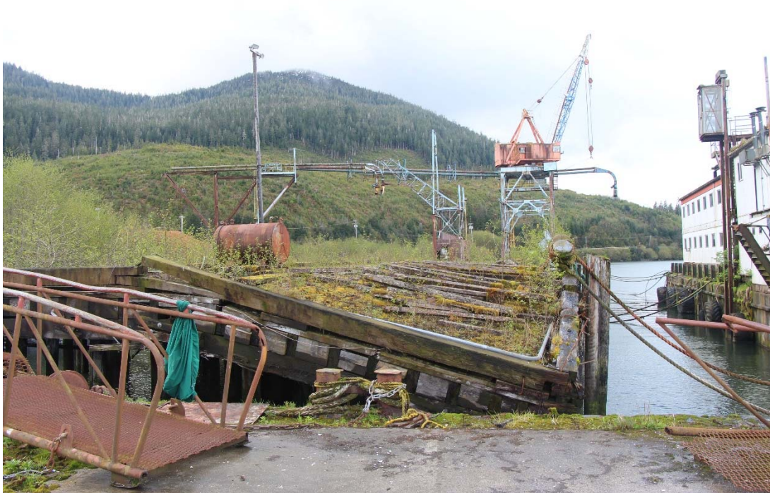
Photo 4 – Damage at North End of Timber Pier
