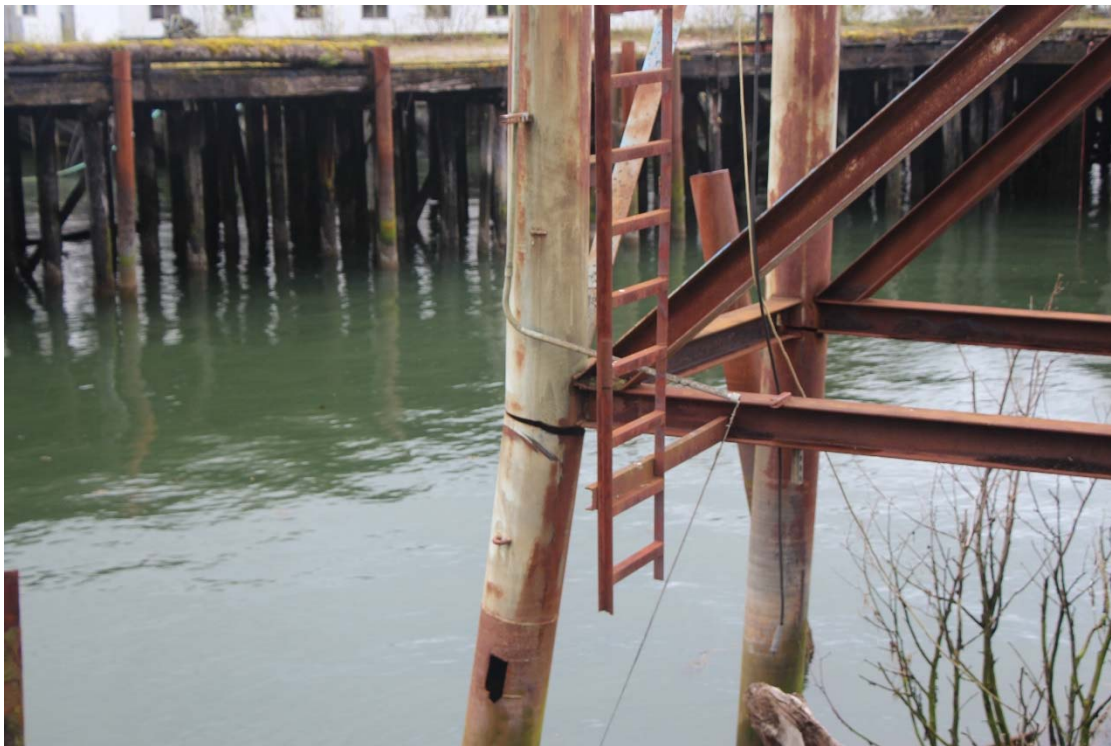
Photo 5 – Failed Column at Shore-side Conveyor Tower
