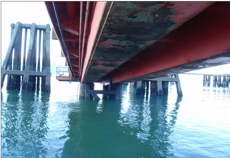
Ramp box-girder bottom flanges; coating failure, minor corrosion, typical.
