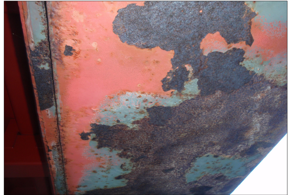
Typical coating failure/corrosion of girder bottom flange.
