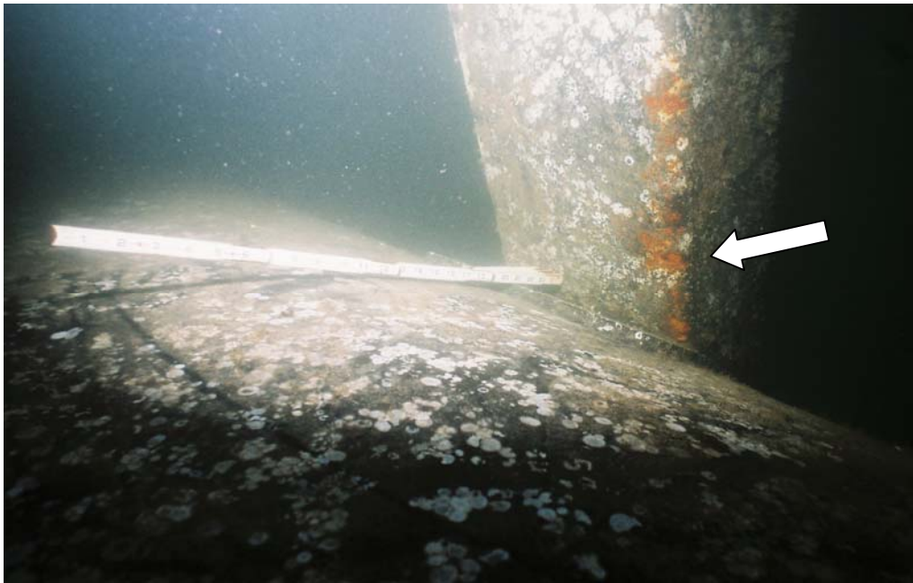
PHOTO No. 9: Seven Foot Diameter Floatation Tank – Note the good condition of the welded connection between the square tubular strut and the floatation tank. Also note the good condition of the epoxy coating on the top of the pontoon and the localized coating failure on the strut.
