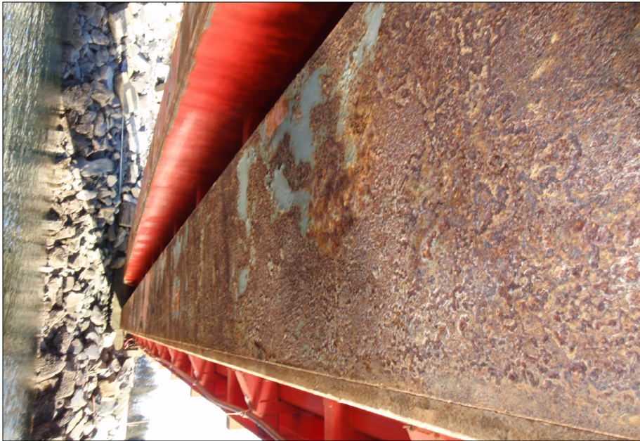
Ramp box-girder bottom flange corrosion.
