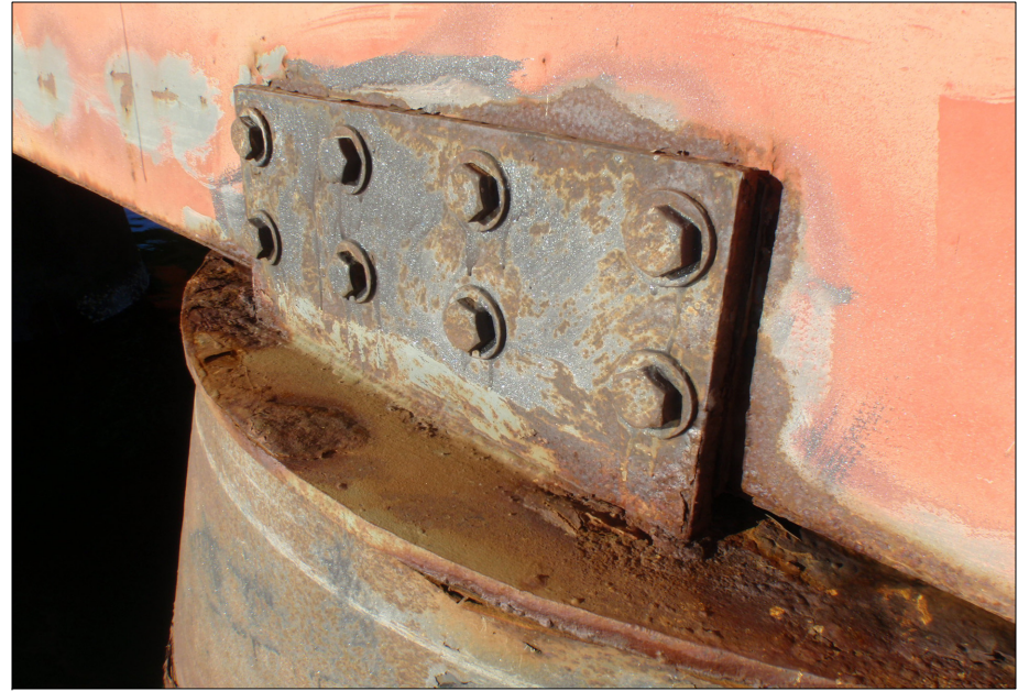
Coating failure/corrosion at ramp/support tank connection assemblies.
