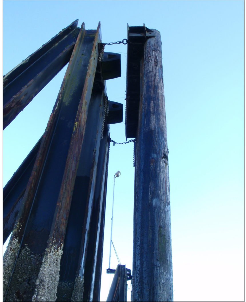
Broken stay chains at Dolphin "C".
