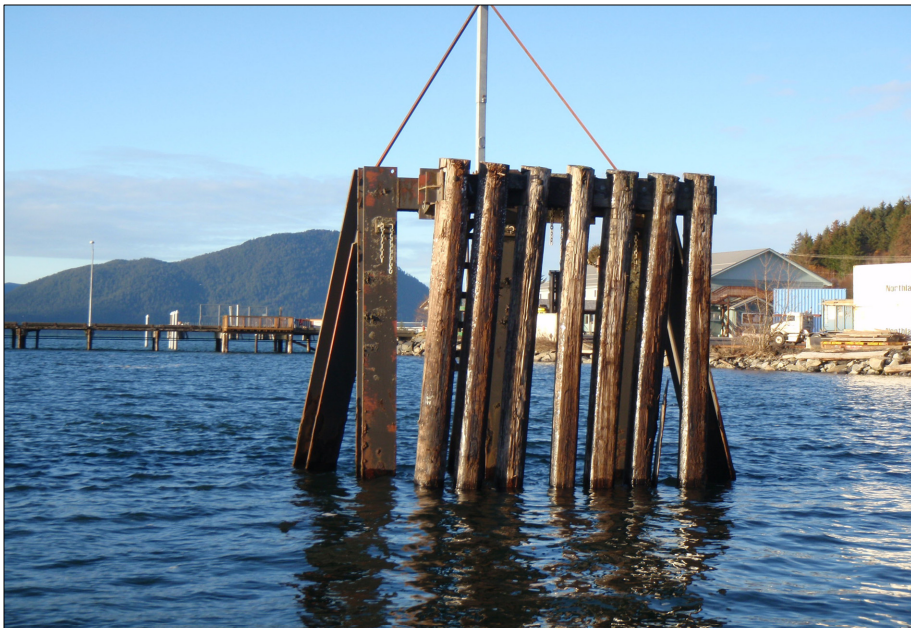
Displaced fender piles at Dolphin "D", looking north.
