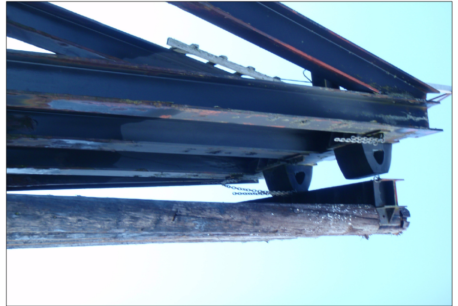
Broken stay chains at Dolphin "D".
