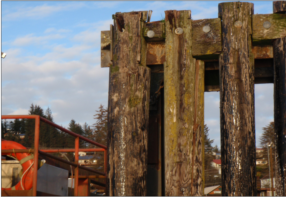
Broken fender pile at Dolphin "F".
