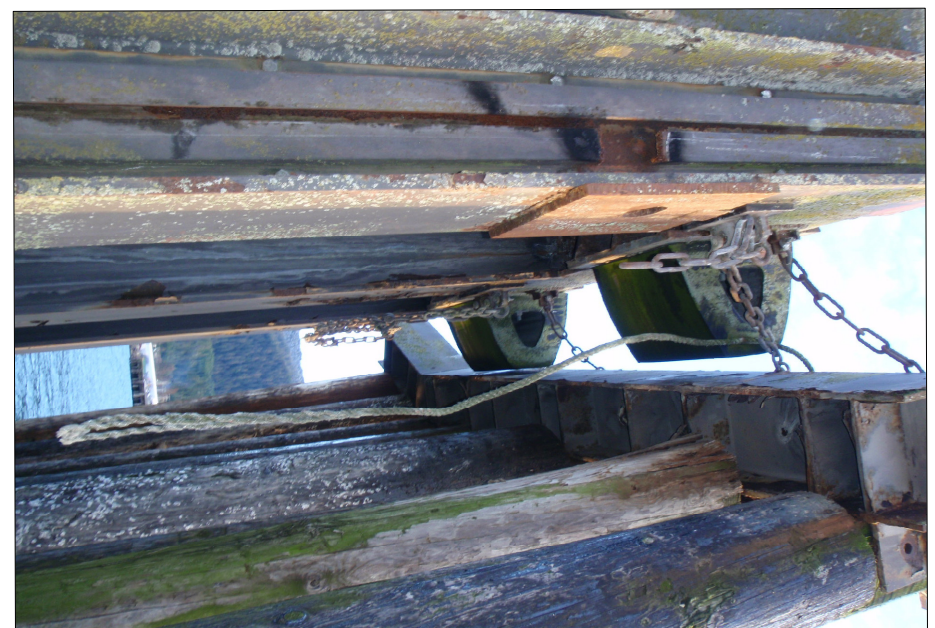
Broken stay chains at Dolphin "F".
