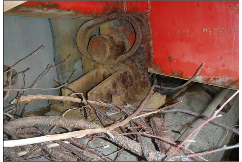
North bearing assembly, debris and worn steel; coating failure on all steel components.
