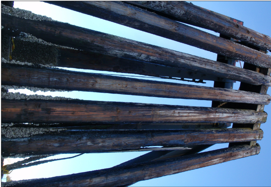
Displaced fender piles at Dolphin "D".
