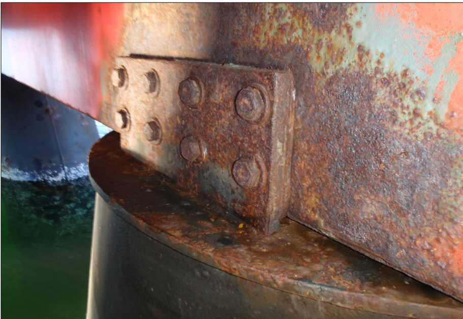
Coating failure/corrosion at ramp/support tank connection assemblies.
