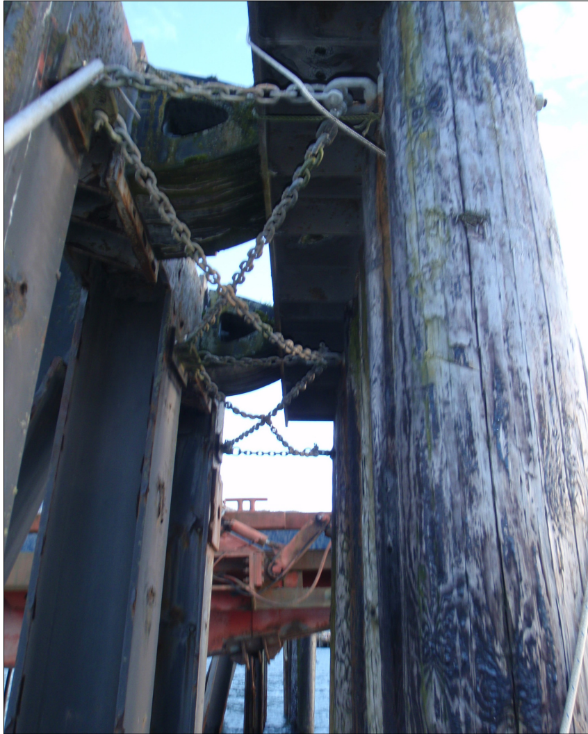
Original stay chain configuration at Dolphin "E".
