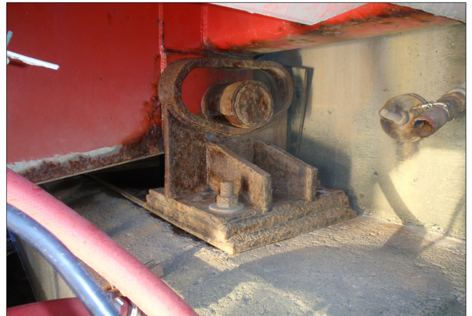
South bearing assembly; coating failure on all steel components.
