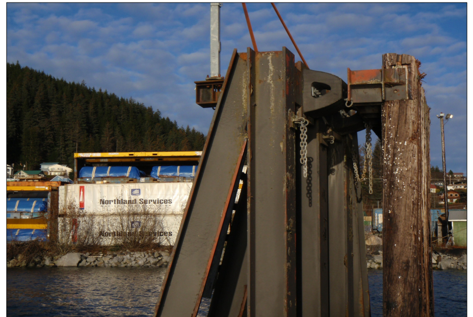
Broken stay chains at Dolphin "D".
