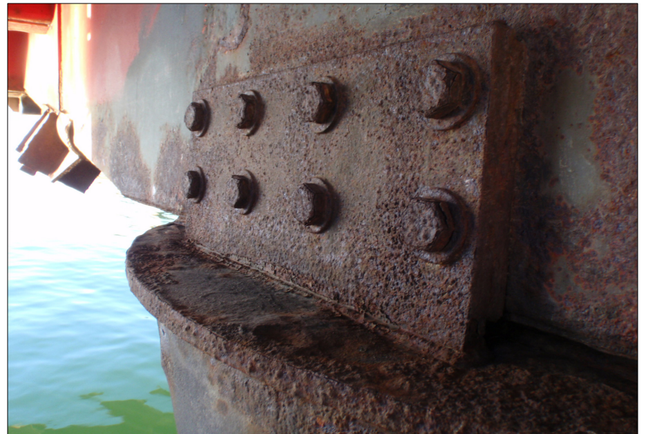
Coating failure/corrosion at ramp/support tank connection assemblies.
