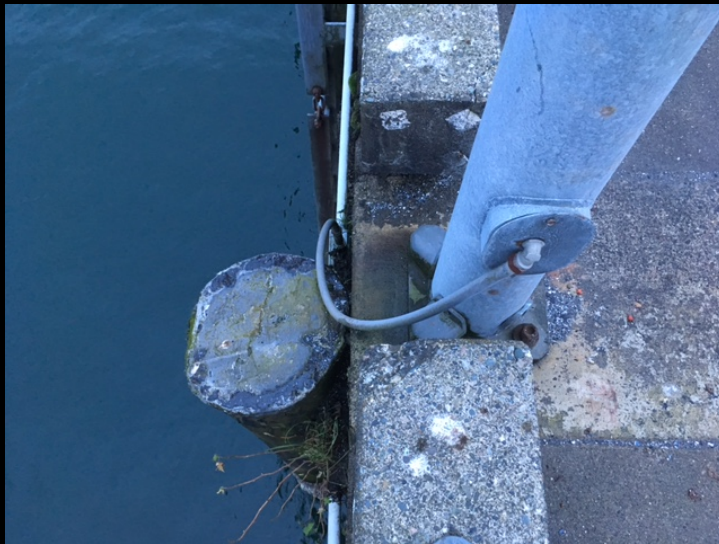
Conduit to Light Pole on Main Dock Lower South End
