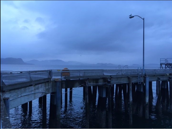
Conduit to Light Pole - Main Dock North End
