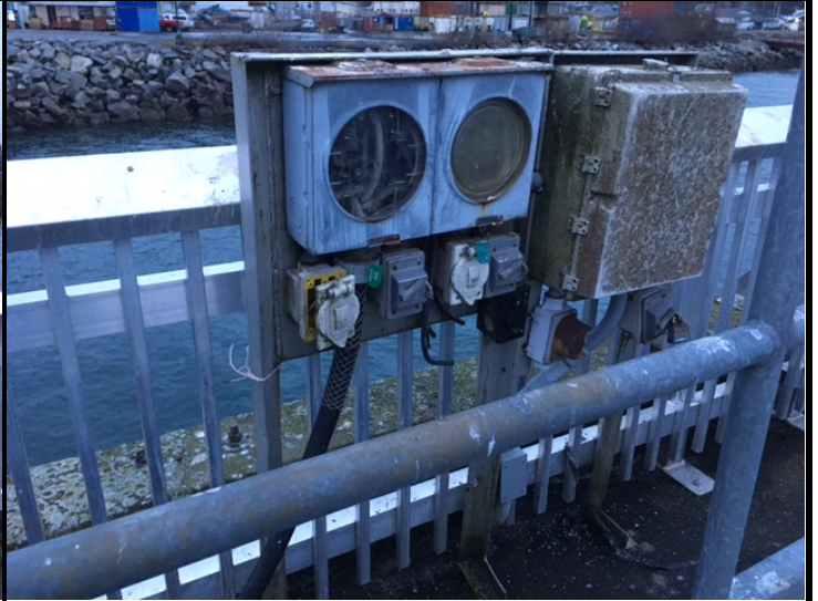
Power Center Equipment on Main Dock
