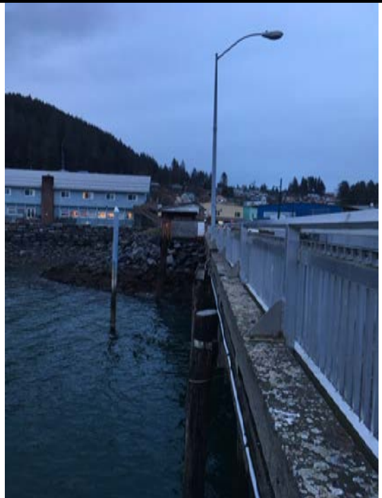
Conduit to Light Pole - Approach Dock North Side
