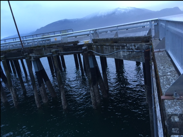
Conduit Along Approach Dock South Side, Turning South Along Main Dock
